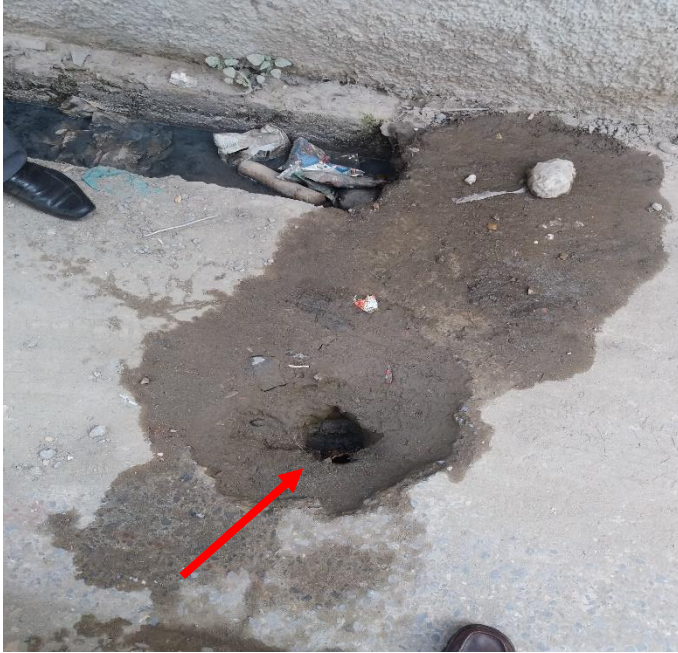
Street valve view in Afshan Colony
