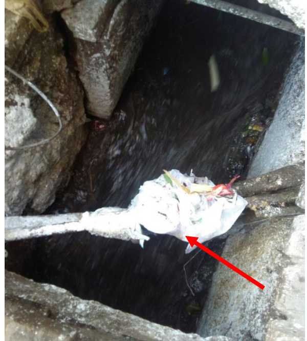
A water pipe crossing across the waste drain at Allama Iqbal Colony
