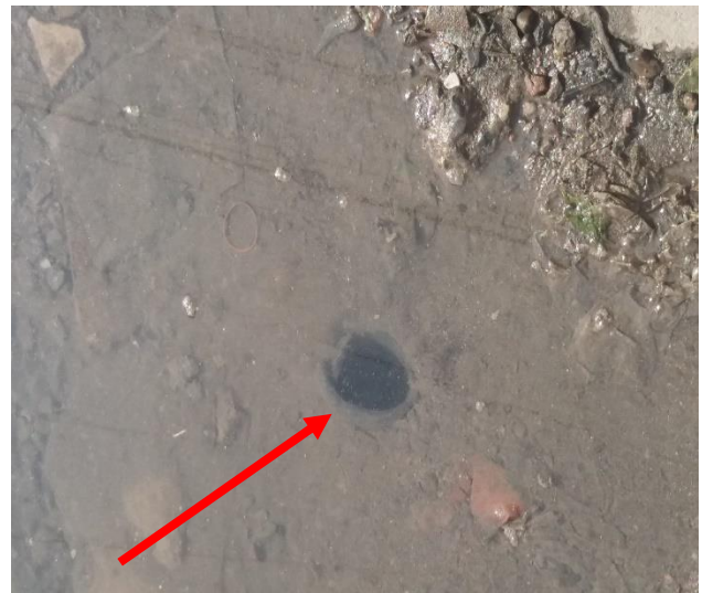
Street valve view in Afshan Colony
