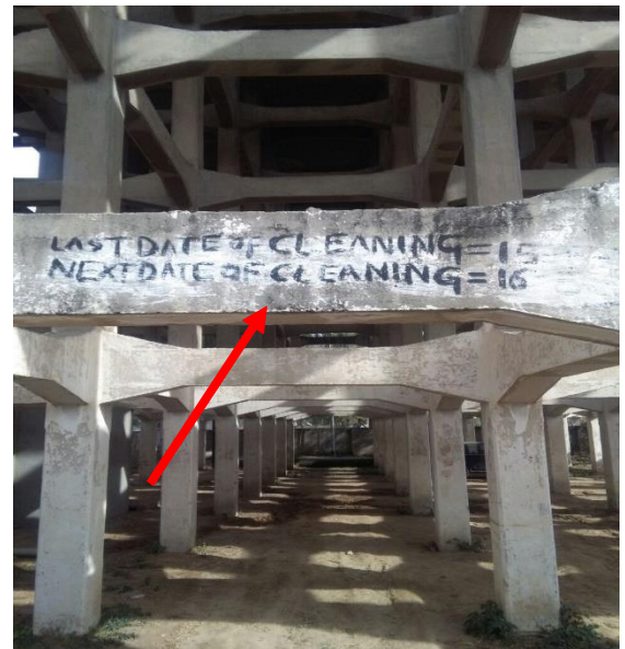
Westridge O/H Tank due for cleaning in 2016
